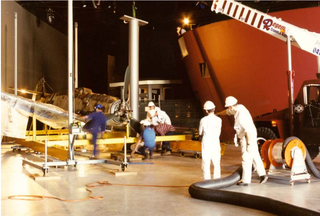
Figure 3. Frontal shot of aircraft in correct position on floor ready for raising. The display support pole is being lifted in with a crane to a position close to the final support site. Note crane exhaust extraction system.
