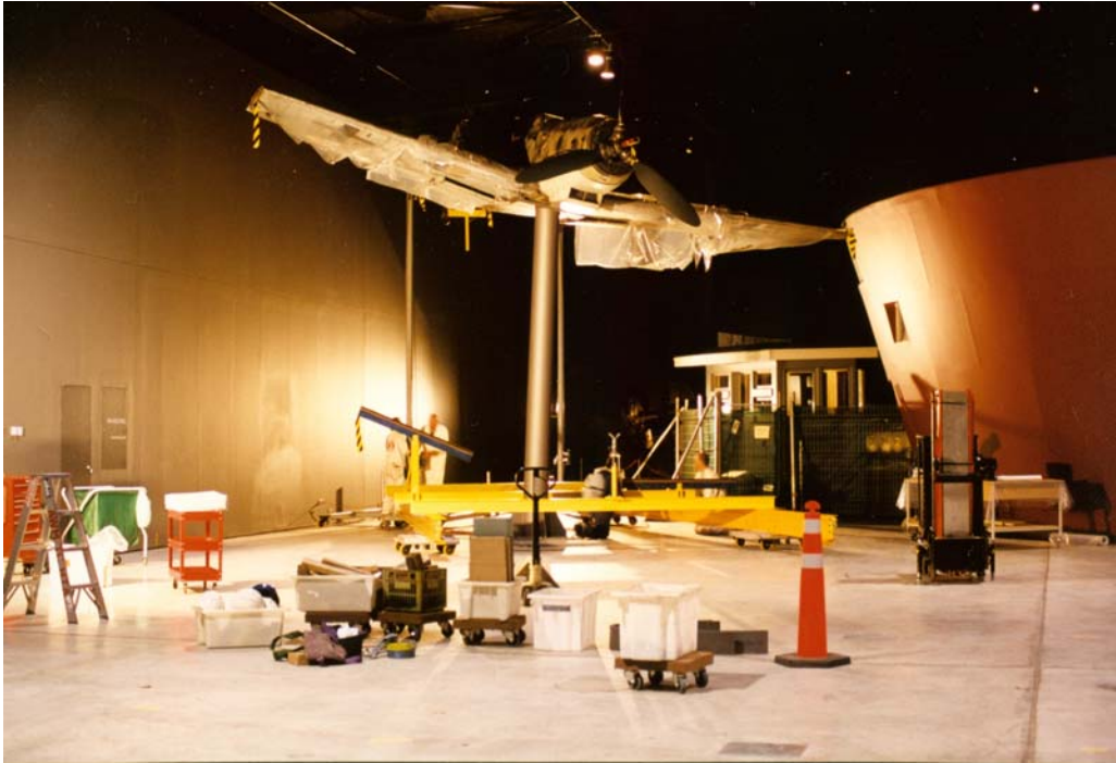
Figure 7. Aircraft installed on support column in final position. Frame has been lowered to the ground for dismantling. Note: the tail support was removed later using a knuckleboom for access.
